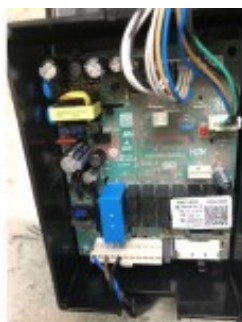
CW 410DT - MAIN PCB BOARD IN ENGINE ROOM (DG3-312) CZE301AZ5000001
